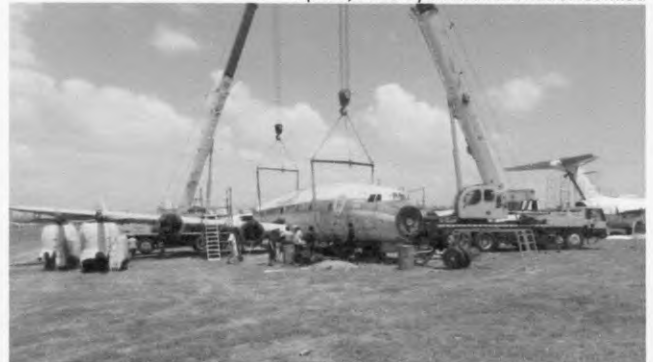
Qantas Founders Museum completes disassembly of Super Constellation ahead of shipment back to Australia
